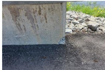
Photo 4: Damage to Concrete Railing Posts
