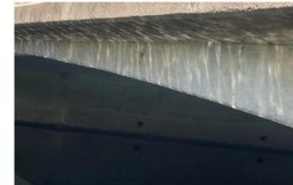
Photo 4: Cracking at Soffit
