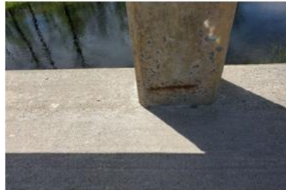
Photo 3: Exposed Rebar at Barrier
