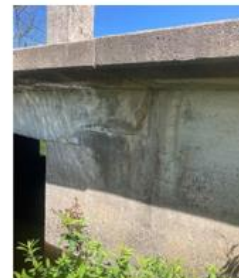
Photo 5: Minor Cracks and Honeycombing Near Bearing Seat
