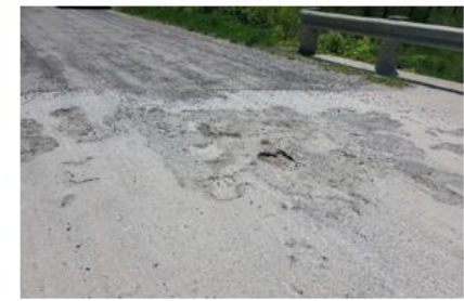
Photo 2: Section Loss at Concrete Deck
