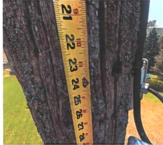
Roof section of Pole exhibiting medium weathering
