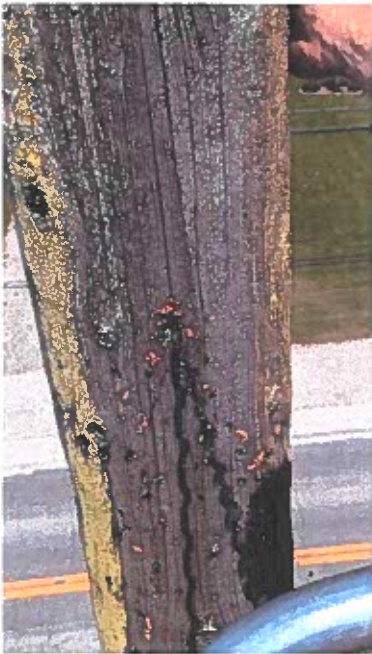
Boring at roof section of right field pole where sounding resulted in a resonant thud indicating a void
