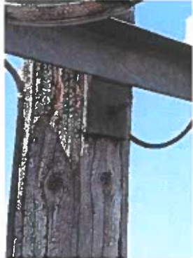
Fixture support bolts exhibit very slight movement indicating fasteners could be re-torqued
