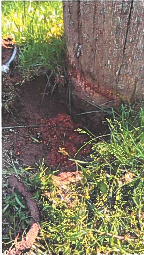
Shell thickness reading conducted at base of left field pole
