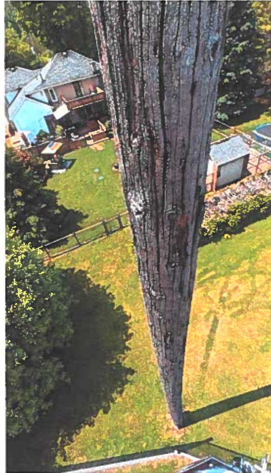
External void exhibiting approximately \frac{3}{4} " Depth 2.5" wide
