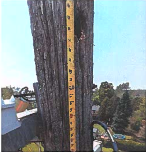
Void at upper roof section of centre field pole
