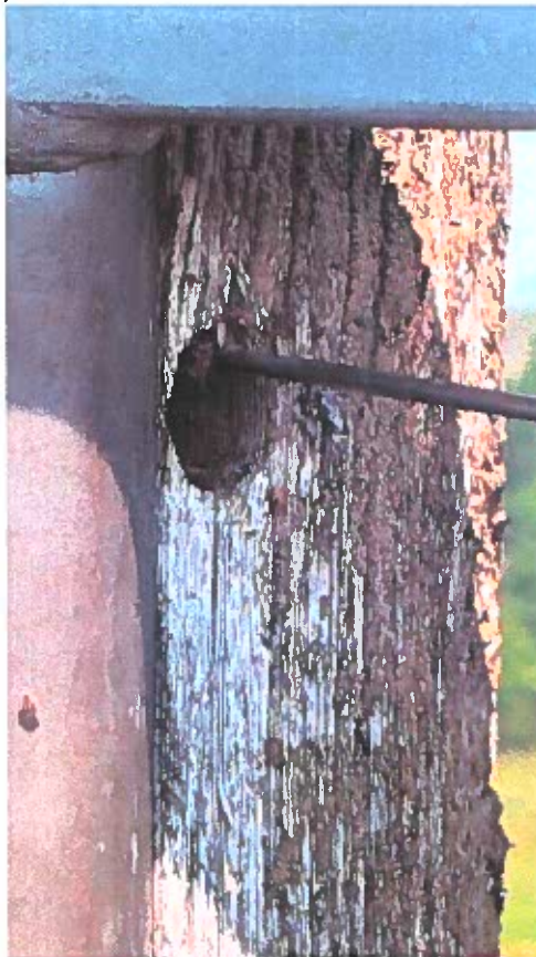
Shell thickness test of upper roof section at old cross arm mounting hole
